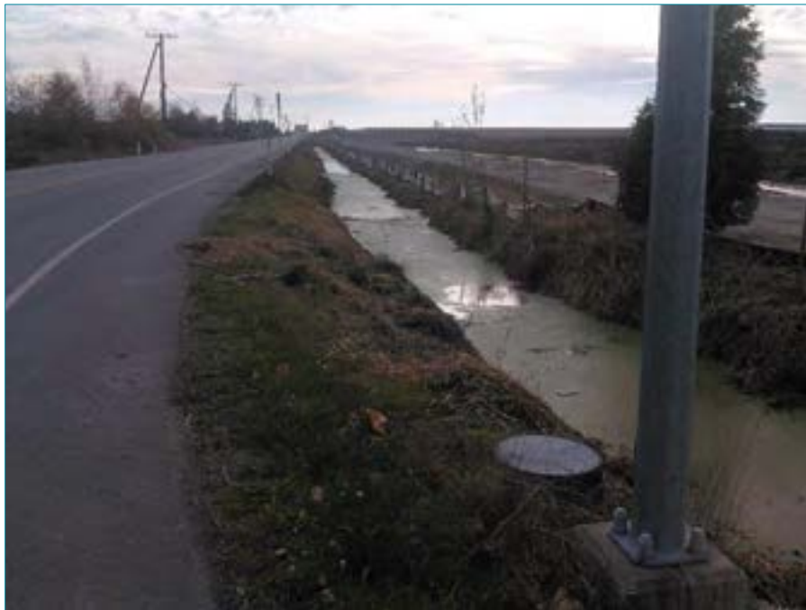
Photo 77: Representative photo of 80 street Ditch West, south of Highway 99 (Watercourse #79), looking south from Ladner Trunk Road. October 17, 2014.
