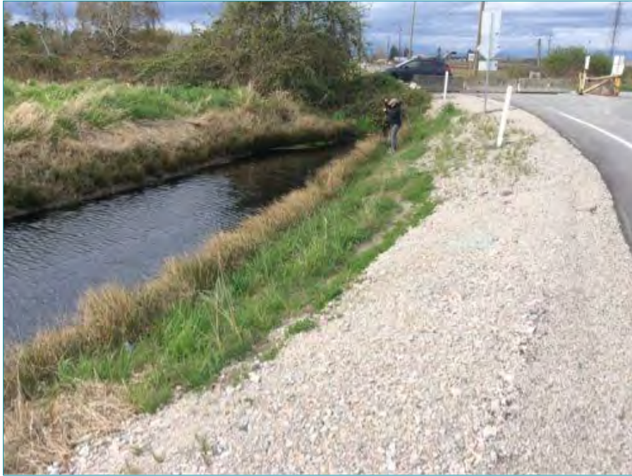
Photo 84: Representative photo of 88 Street Ditch West, north of Highway 99 (Watercourse #88), facing north. April 15, 2014.
