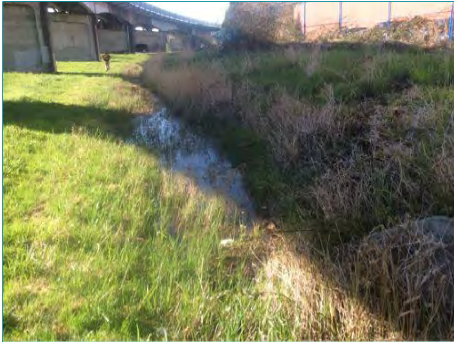
Photo 1: Swale that runs to the north from Bridgeport Road North (Watercourse #6), looking south. April 1, 2014.
