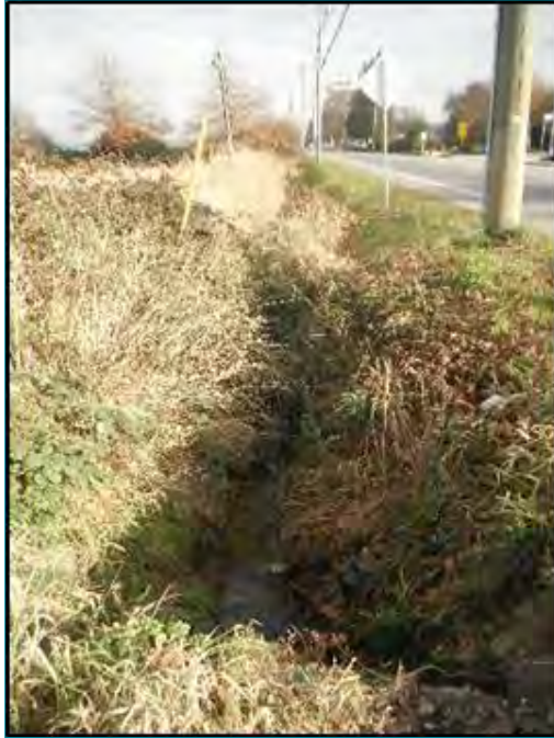
Photo 96: View of Ladner Trunk Road Ditch North, east of 96 Street (Watercourse #100), facing north from Ladner Trunk Road. October 18, 2014.
