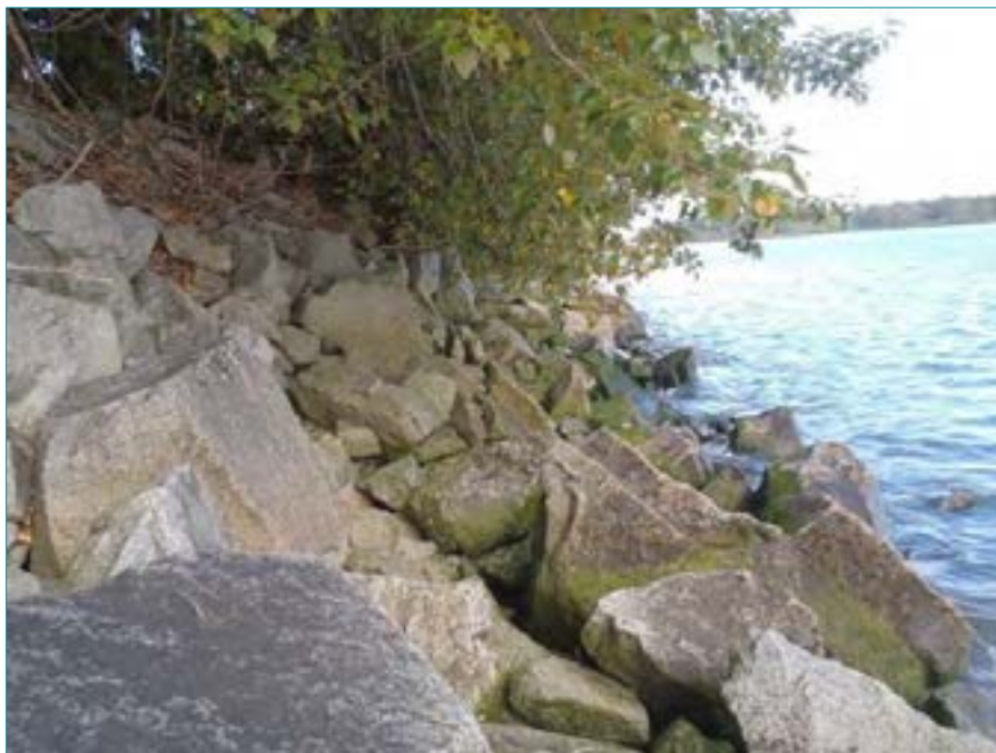
Photo 46: Riprap armoring on intermittent sections of River South Arm south bank. February 19, 2014.
