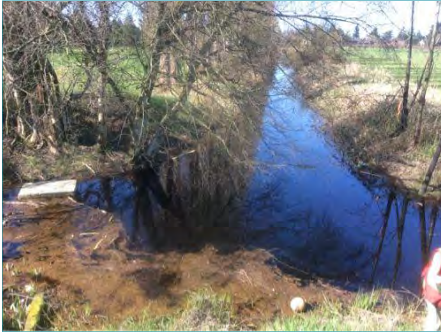
Photo 27: Looking west from Highway 99 at King Road Ditch, west of Highway 99 (Watercourse #33). April 1, 2014.
